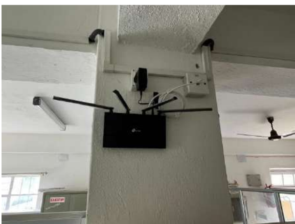
5. 01 no. of Wi-Fi Router installed at Teaching Staff Room, SGC, Rhenock.
