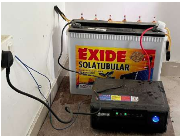
12. Inverter system installed for uninterrupted power supply at Commerce Block, SGC, Rhenock.
