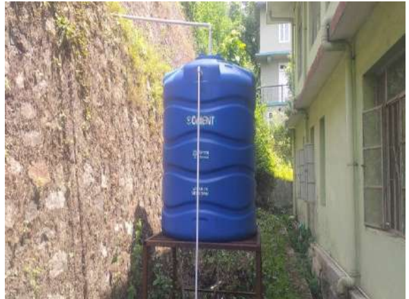
16. Line distribute at Administrative Block.
