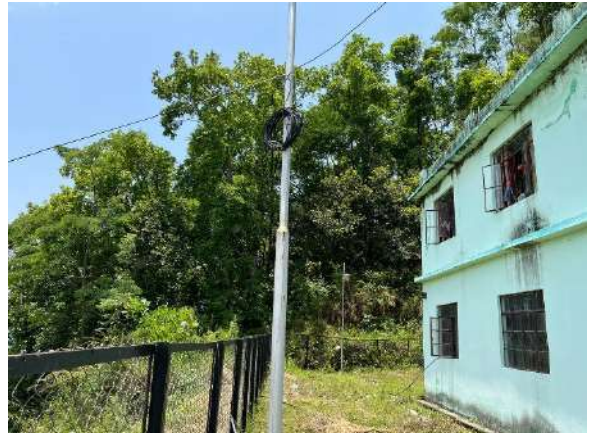
27. For support of 6 OFC Wire, Iron pole installed at Girls' Hostel, SGC, Rhenock.
