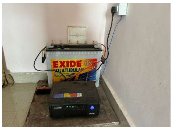
15. Inverter system installed for uninterrupted power supply at Principal Quarter, SGC, Rhenock.
