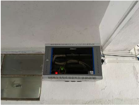
8. 6 U Rack Fully Loaded installed at Academic Block, SGC, Rhenock.
