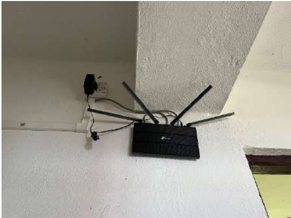
26. 01 no. of Wi-Fi Router installed at Left Side of 1 st Floor, Girls' Hostel, SGC, Rhenock.
