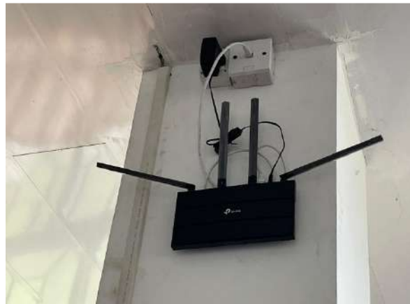
4. 01 no. of Wi-Fi Router installed at Library, SGC, Rhenock.
