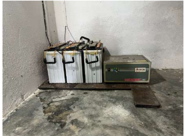
23. Inverter system installed for uninterrupted power supply at Girls' Hostel, SGC, Rhenock.
