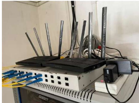
2. Main Routers for supply of 80 MBPS Internet connectivity from Exchange to SGC, Rhenock.
