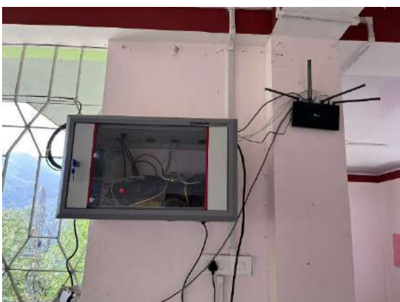
14. 6 U Rack / 01 no. of Wi-Fi Router installed at Principal Quarter, SGC, Rhenock.
