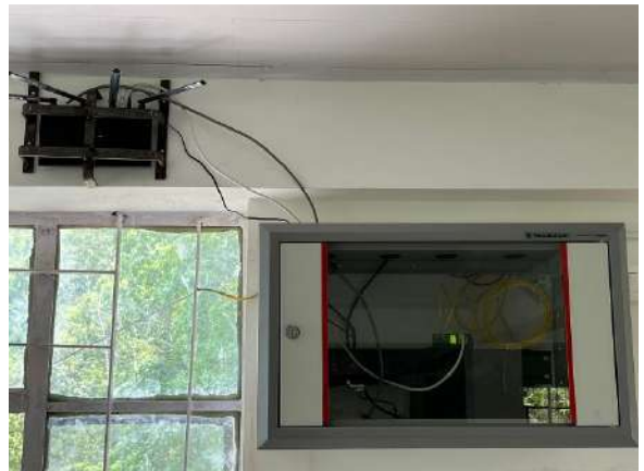
11. 6 U Rack / 01 no. of Wi-Fi Router installed at Commerce Block, SGC, Rhenock.
