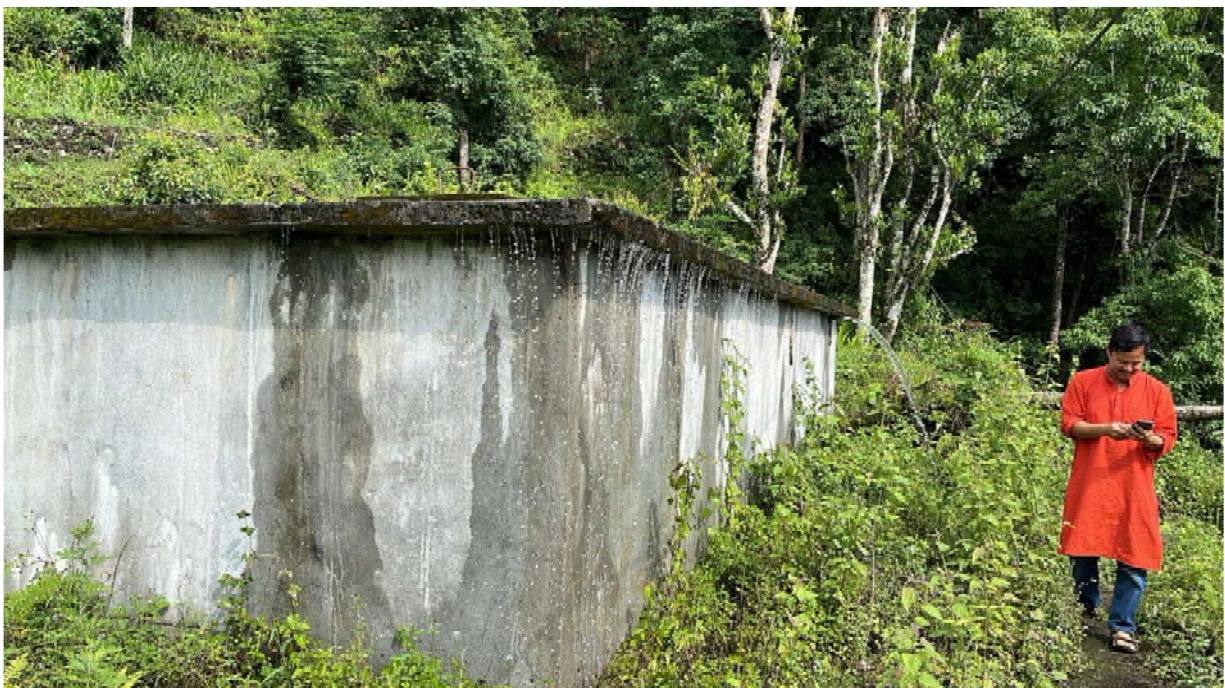
17. Main water reserve tank of Sikkim Govt. College, Rhenock
