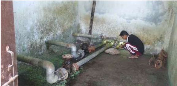
1. Main Line connecting and valve fitting at Chalampong WTP, PHE clear water reserve tank.
