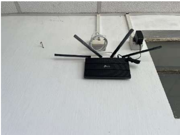
10. 01 no. of Wi-Fi Router installed at Right Side of Top Floor, Academic Block, SGC, Rhenock.
