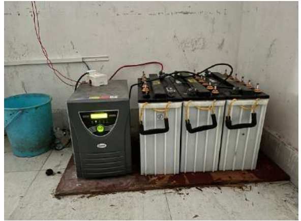
9. Inverter system installed for uninterrupted power supply at Academic Block, SGC, Rhenock.
