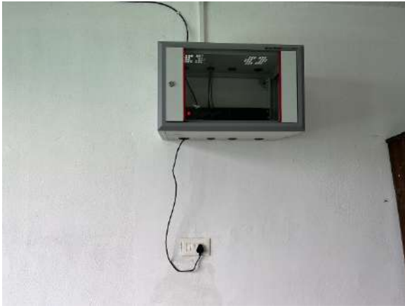
22. 6 U Rack installed at Girls' Hostel, SGC, Rhenock.
