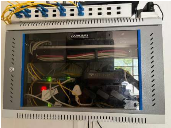
1. Main 6 U Rack Fully Loaded installed at Administrative Block, SGC, Rhenock.
