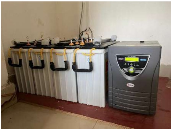
3. Inverter system installed for uninterrupted power supply at Administrative Block, SGCR.
