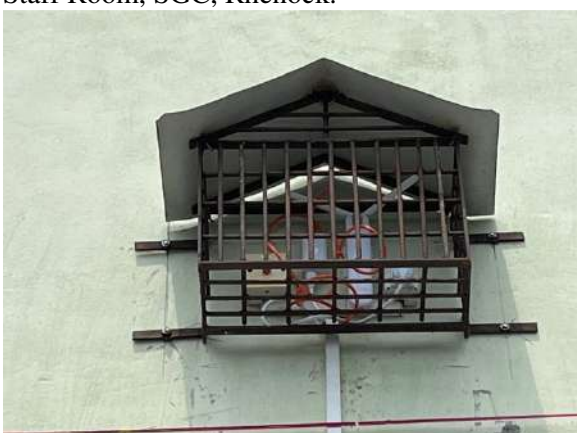
7. 02 nos. of Outdoor Wi-Fi Router installed at Academic Block, SGC, Rhenock
